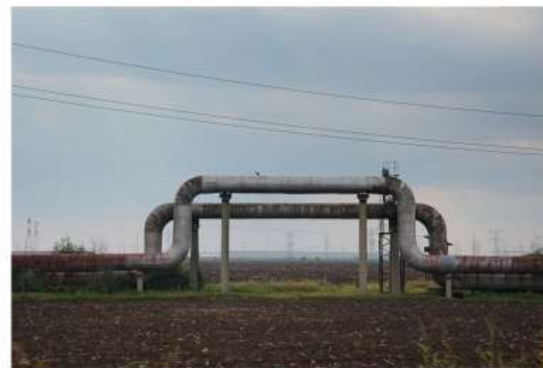
A TRACTOR GATE FOR AN OIL PIPELINE IN ROMANIA. PHOTOGRAPH BY PEPSEBNU, LICENSED UNDER CC BY-SA 3.0
